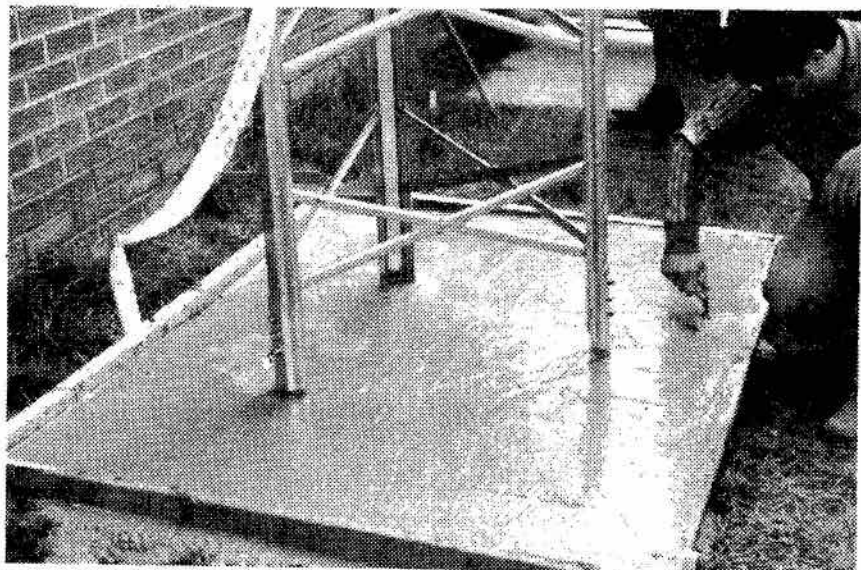
Leon VE2 DTH putting the final touch on the newly poured cement.
