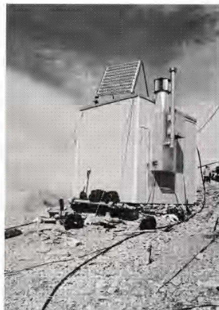
The building that houses the VE6HWY repeater. Note the solar panels on the roof. That's the helicopter in the background. ■
